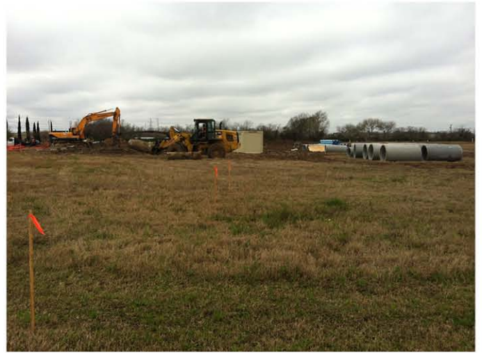
Photo 2: South portion of the site where infrastructure for this phase and the surrounding area are being constructed and installed.
